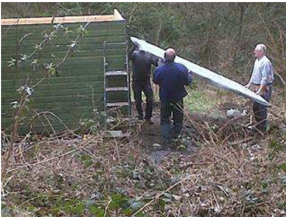
Bryan, Paul Lythgoe and Paul Heaton put the roof on the hide.
